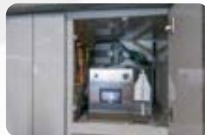
ADS mounted on cabinet shelf
