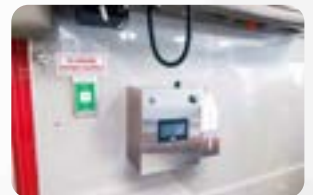
ADS mounted on compartment wall
