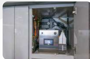
ADS mounted on cabinet shelf
