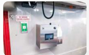
ADS mounted on compartment wall
